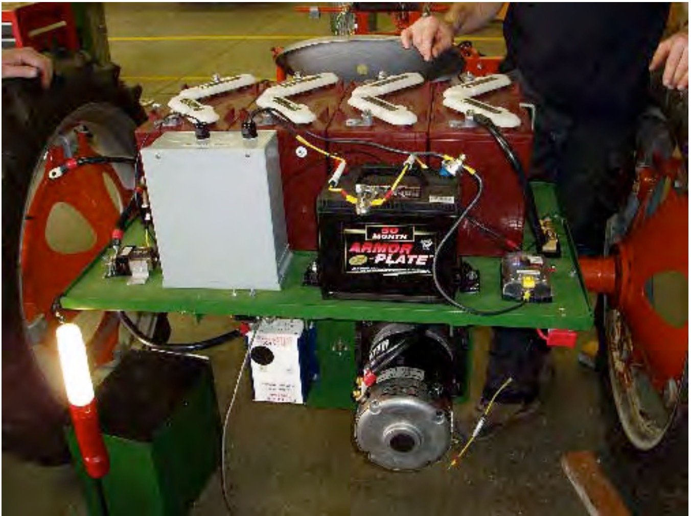
Battery rack and battery bank installation.
